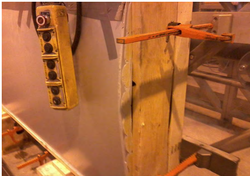
Photo No. 2 ACM Panel System (Wet Seal) Mode of Failure
